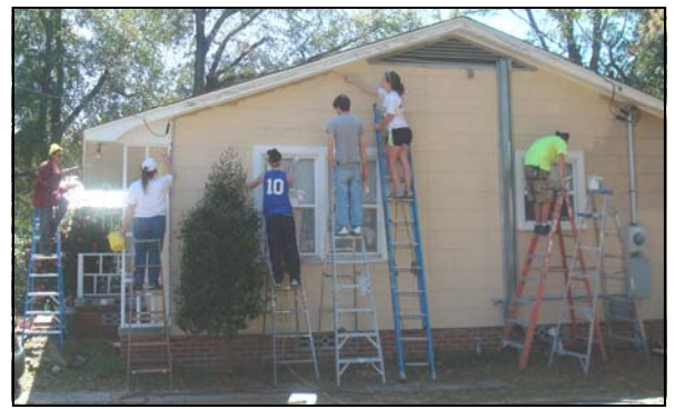
We love ladders, paint and safety (does everyone have 3 points of contact at all times?)
